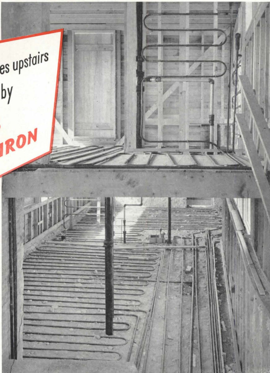
BENNETT RESIDENCE—BARRINGTON, ILL. George F. Keck, Architect John Fairbairn, Engineer Illini Heating Co., Contractors and Fabricators
