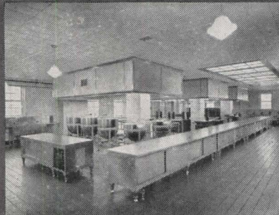
MAIN KITCHEN. Completely Monel-equipped by The John Van Range Company of Cincinnati, Ohio.
