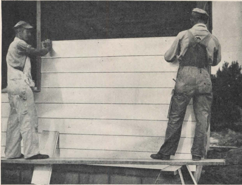
Reynolds Lifetime Aluminum Clapboard Siding going up on a typical veteran's home. Note the precision of line — with no leveling off. Note the butt joint, on the fourth clapboard from the top.
