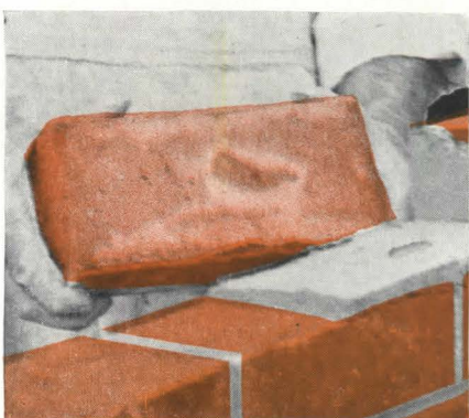
Therefore the mortar did not stick to the top brick. A good bond was not secured.
