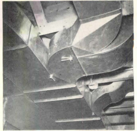
Aluminum ducts for heating or ventilating
