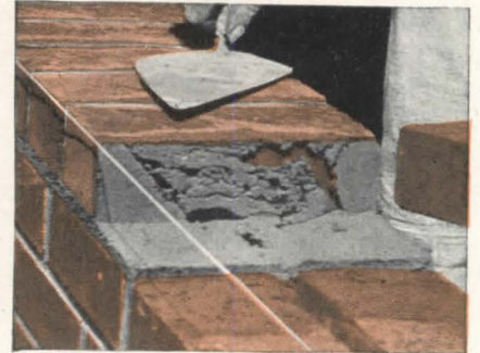
Slushing will not fill the voids.
