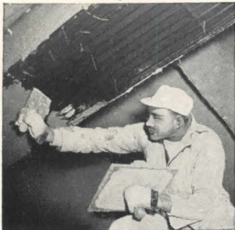
PUT ON THE PLASTER! Note the Monel Tie Wires holding this steel screening in place. Monel resists corrosion by alkalis and salts in plaster, lime and other building materials.
