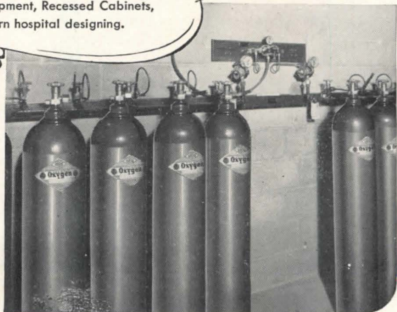
CENTRAL OXYGEN PIPING SYSTEM
