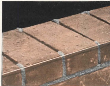
there is nowhere near enough mortar in the joint.
