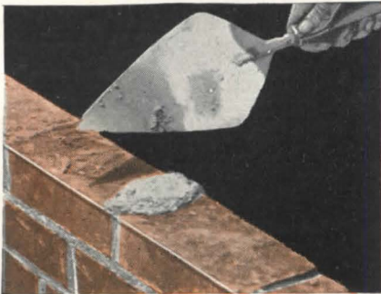
Slushing does not properly fill the voids in the head joints.
