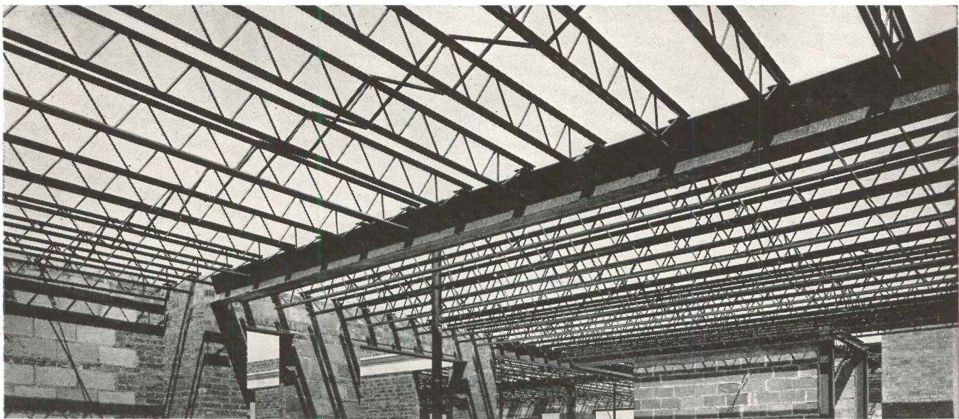
Construction scene, taken during erection of apartment buildings above, showing Bethlehem Open-Web Joists in place.
