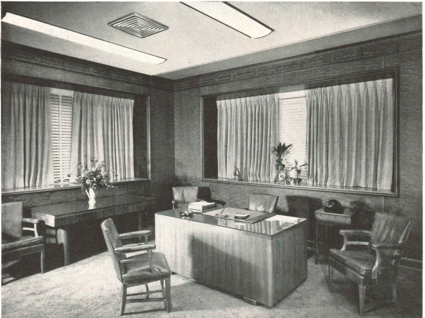
Air diffusion beauty and efficiency is achieved with Agitair Type R in Presidents Office, City National Bank
