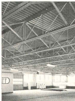
Truscon "Clerespan" Joists in Heindel Oldsmobile Garage, Youngstown, O.
