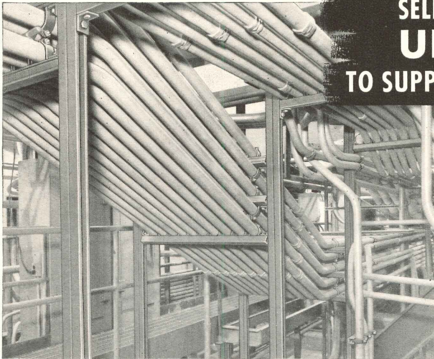
Heavy rows of conduit are quickly installed and easily supported with completely adjustable Unistrut channel, fittings and clamps. Note examples of combination racking where conduit is clamped above and below to channels mounted back to back.
