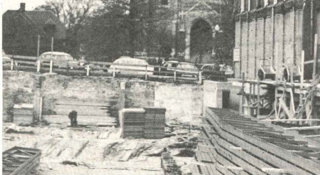
Truscon "Clerespan" Joists were used to obtain large unobstructed areas in the Star Market, Newtonville, Mass.
