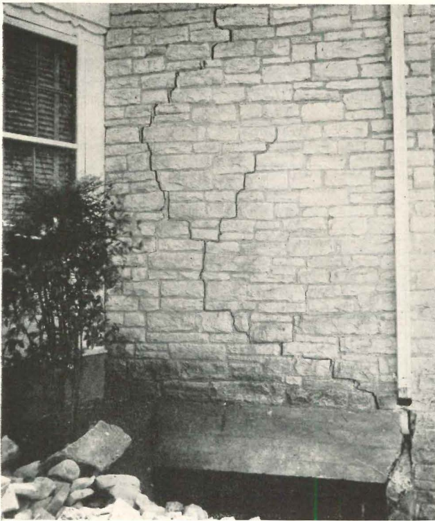
1. Expanding clay soil caused the enormous cracks in this wall
