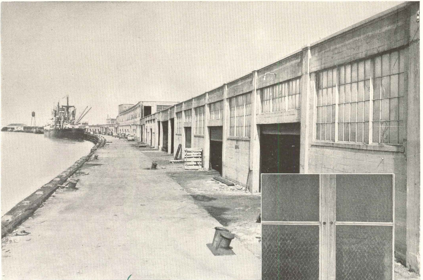
Partial view of the galvanized, unpainted Fenestra Steel Windows in the huge Mallory Pier of the Galveston Wharf Company, Galveston. And here is an unretouched closeup of one of the unblemished windows after a 23-year-long test of salt spray.
