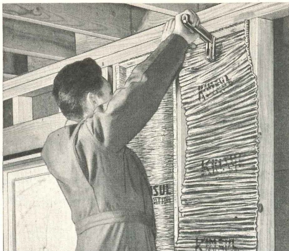
1 Required length of KIMSUL* blanket is cut from roll and stapled to top plate through fiber strip.
