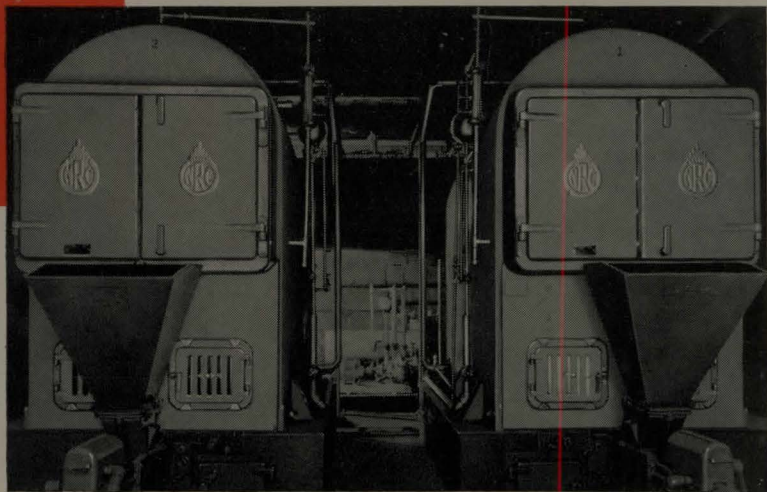
View of the two No. CA-6630 NATIONAL Commercial Steel Boilers with stokers in the Monongahela High School, Monongahela, Pa. Myers & Myers, Monongahela, Pa., Heating Contractors.
