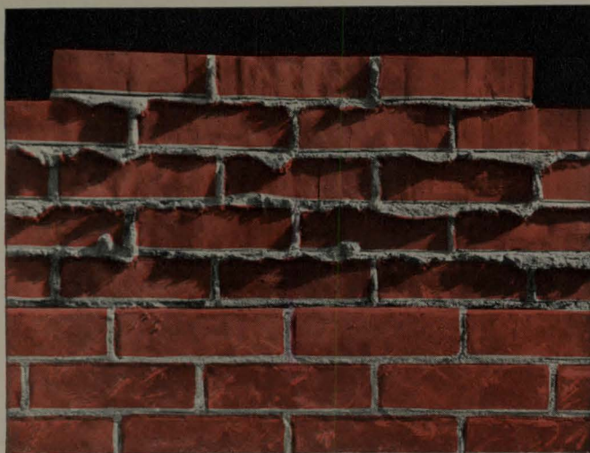
Backplastering should not be attempted over protruding mortar joints.
