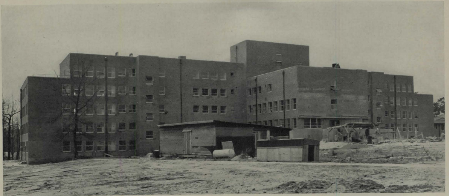
Mississippi adds 166 beds to its program for controlling tuberculosis among its negro population with this infirmary, shown here in construction views, an addition to an existing institution. Upper view shows principal facade, facing south
