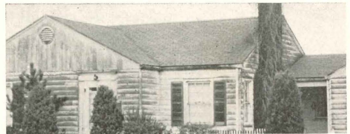
2 Paint has eroded by excessive chalking causing failure. Since paint has chalked off the unheated garage (right) as well as heated house walls, improperly formulated paint is the trouble rather than condensation behind the wood
