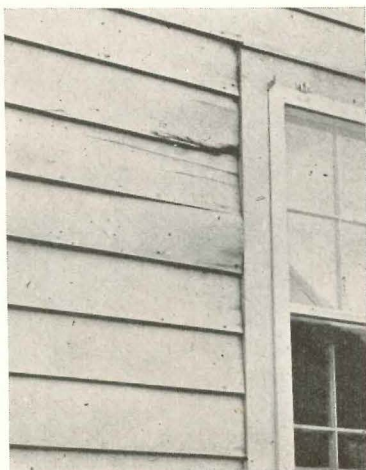
1 Durable paint will not correct this construction defect. Wood siding has rotted around improperly flashed window opening. House was painted four years before this photo was taken
