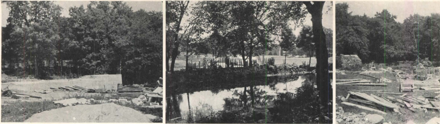
Three Chapels under construction: the pool glimpsed in center photograph is central in site plan (opposite)
