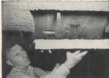
FIBERGLAS insulation, Type PF-613, 2" thick — bonded to concrete ceiling using MIRACLE PRONGED ANCHORS at Radio City Studio 6B, New York, N. Y. CONTRACTOR, William J. Scully, Inc., New York, N. Y.
