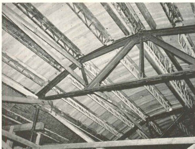
Five forms like this were used for pouring the 93-ft shells in three sections. Forms were built well because of future need
