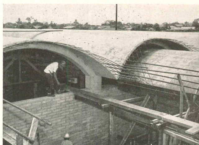
The form is being positioned for one of the three 32-ft barrels. Reinforcing steel projects to make a tie with the 93-ft shell
