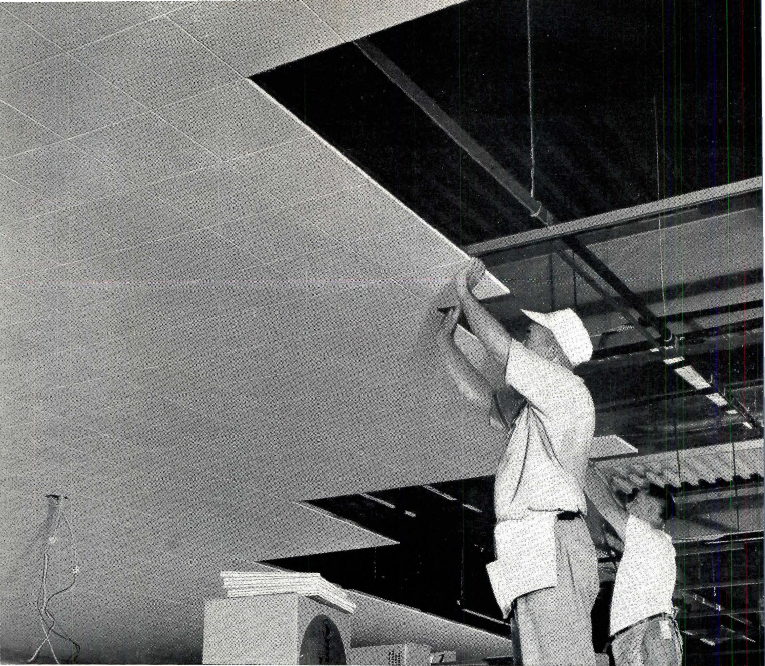
These mechanics are installing an Armstrong Minatone Ceiling under ideal job conditions. Electrical work has been located, and the building is thoroughly dry.
