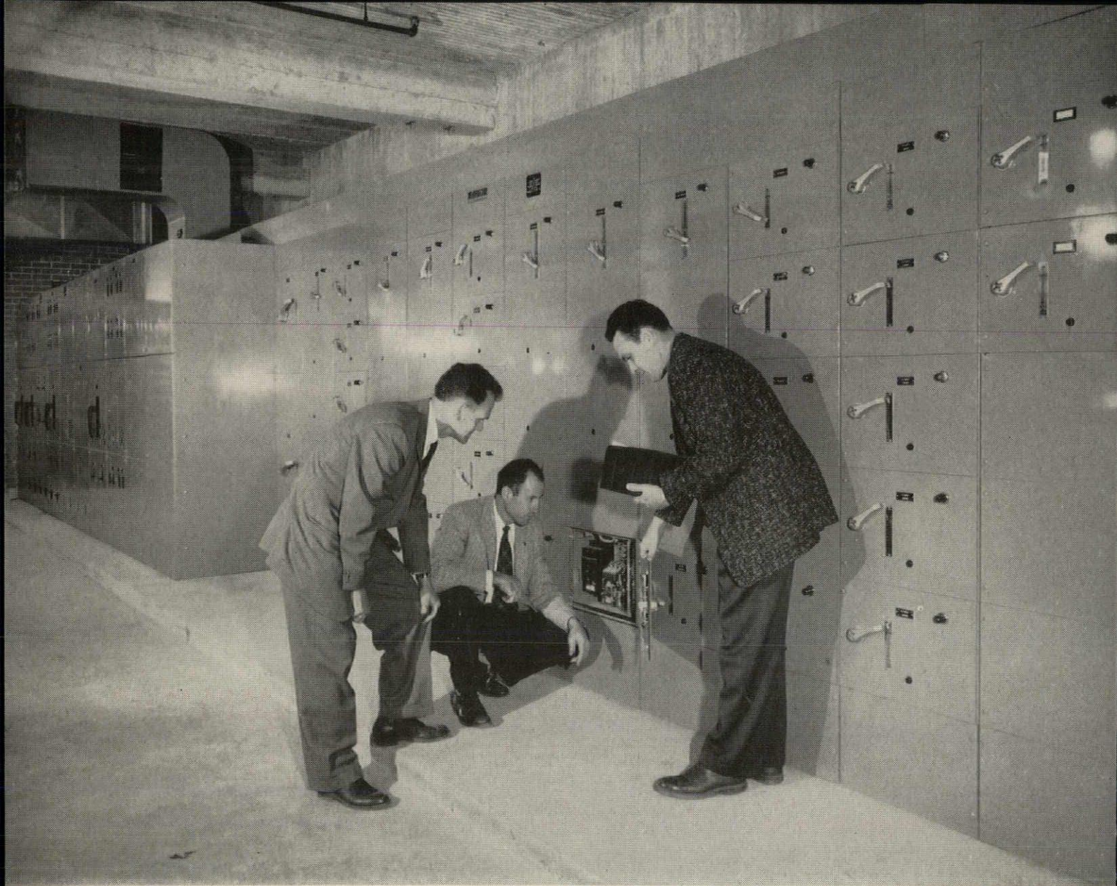
Gerald B. Smith and Max Waddoups look into cubicle of Westinghouse control center as Don Black reviews specifications. This control center and building type switchboard provide centralized control and protection of all important lighting feeder and motor circuits.
