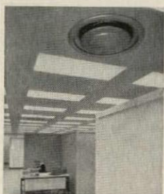
A standard Kno-Draft diffuser in an office area.
