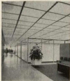
In grid ceiling areas, diffusers and return registers are entirely hidden.
