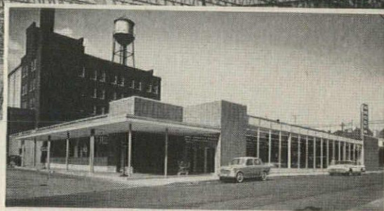
Kroger Supermarket, Charleston, W. Va. 145 x 140 foot wall bearing V-LOK frame. Upper photo shows framing completed—only 5 days after delivery of steel.
