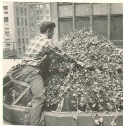
Workman spreading ivy runners out conically between planting boxes to give an immediate finished effect. Next, ivy was attached to wire mesh to prevent it from being blown out of position
