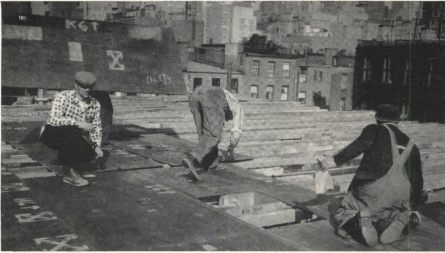
After setting up column forms and framing for decking, workmen lay plywood deck forms for flat plate slabs. Markings indicate the position of each panel, as well as the location of each break in the slab. Three sets of forms, all identically marked, were used on the job, requiring only verification of markings as each floor was formed
