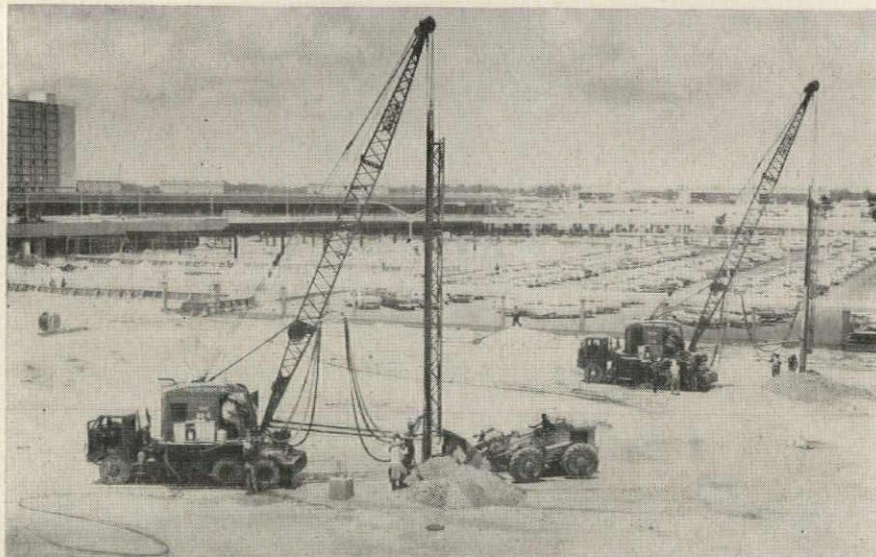
Vibroflot machines compacting sand foundation to a depth of 20' for new 2-level, 5-acre parking deck between the airport's entrance ramps. Architects: Steward-Skinner Associates; Consulting Engineer: William H. Weaver; General Contractor: Fred Howland, Inc., - all of Miami, Florida.
