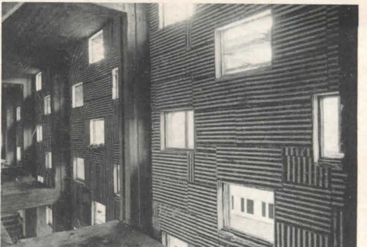
Figure 4. Polystyrene foam on the walls of a swimming pool hall supports the plaster and provides thermal and condensation insulation
