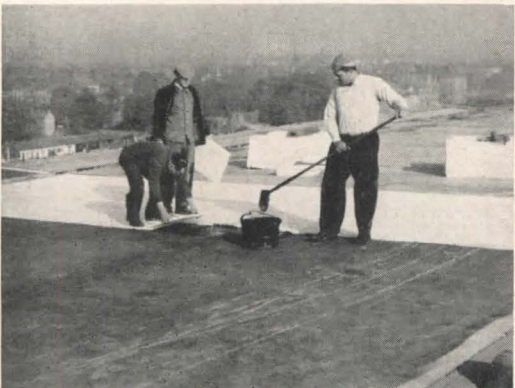
Figure 6. The roof is built up in the usual way after the polystyrene foam has been covered with a layer of asphalt-coated paper
