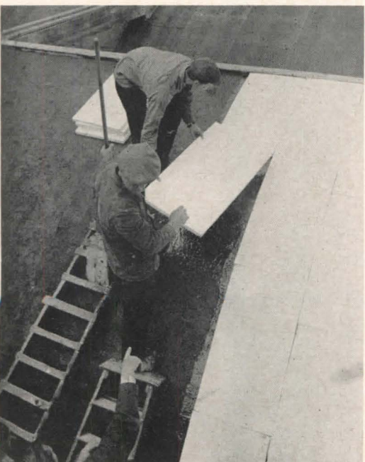
Figure 7. Polystyrene is used similarly on sloping roofs, but if the roof is wood, it is applied from beneath and supported on a lattice
