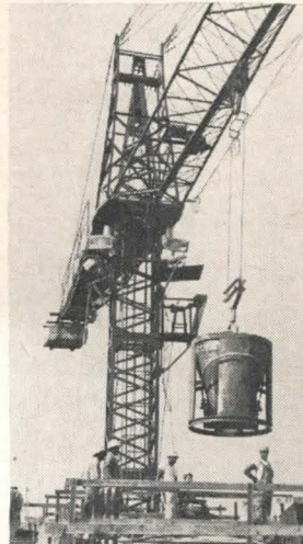
Crane is remote-controlled by one man from working deck with 3½ lb. electronic panel. He is free to move to any part of the job, and to assist in loading and unloading.
