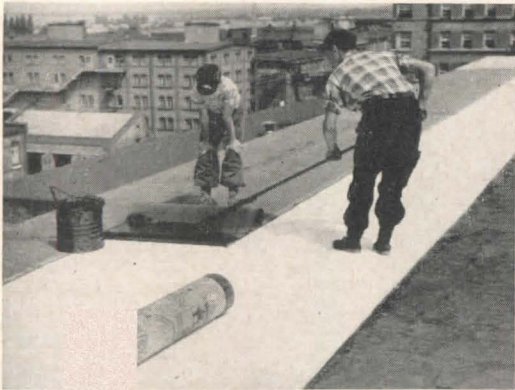
Figure 5. On flat roofs, insulating polystyrene foam sheets are laid on top of a layer of hot asphalt applied over a dry asphalt emulsion
