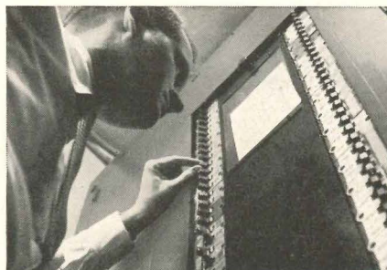
Old system controlling corridor lights required manual operation of panel switches on 33 floors. A half-hour job!
