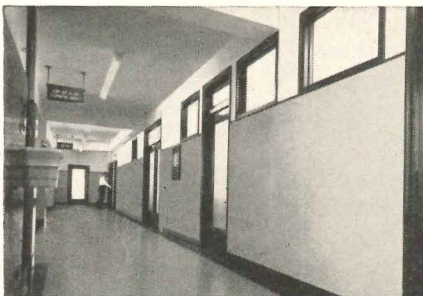
Each corridor has two sets of controlled lights — one ON every day — one near windows, ON when its dark outside.
