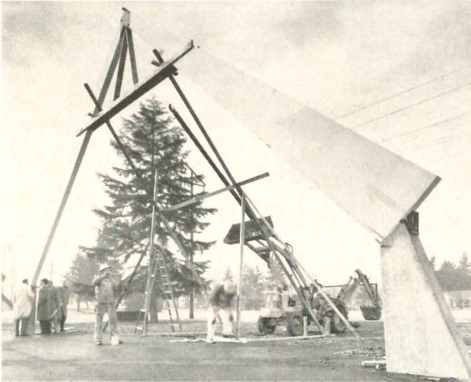
The structure shown above is the DFPA-built prototype of the "delta frame," a rigid bent composed of two tapered box beams with additional tapered box beams cantilevered from each side. The photo above left shows the first of the
