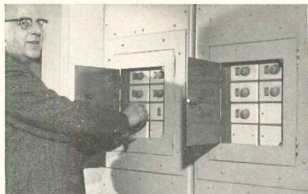
G-E master selector switches at ends and center of each floor control lighting separately for each 1/2 floor. Building contains 2000 fluorescent lamps.
