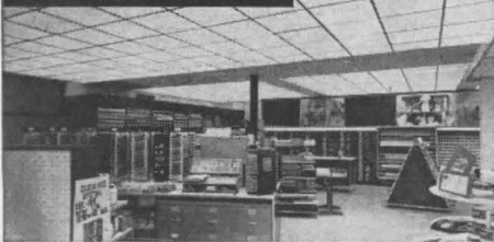
Circlgrid Luminous Ceiling installed in retail store
