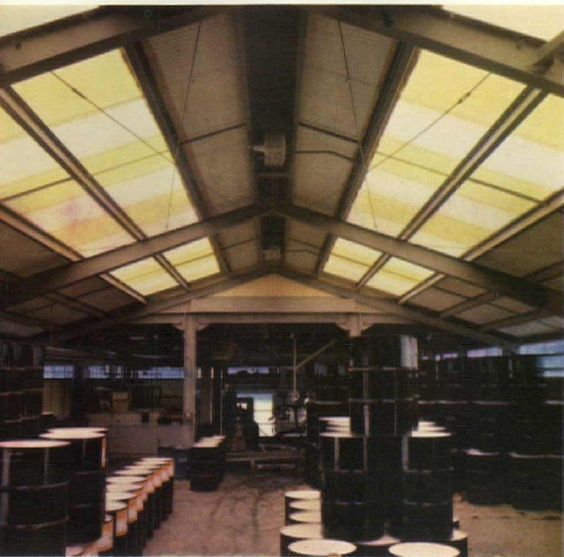
Panels resist fumes in Baton Rouge chemical plant.
