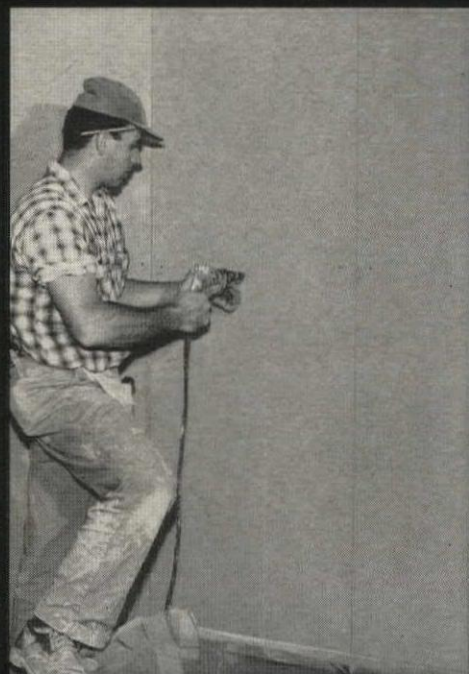
E. Screw face panels to gypsum coreboard on each side of double-wall partitions
