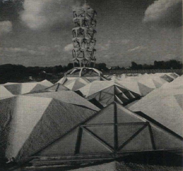
Tower is the work of sculptor Robert Cronbach. It is positioned over the beam in the sanctuary. Precast Star of David units and skylights make curious roofscape
