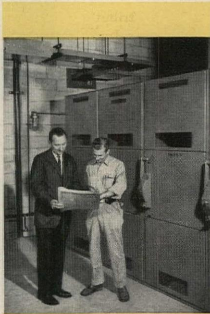
This installation of Square D unit substations transforms the 13,200-volt incoming power to 480-volt utilization voltage. The totally enclosed feeder duct overhead carries power throughout the Center.
