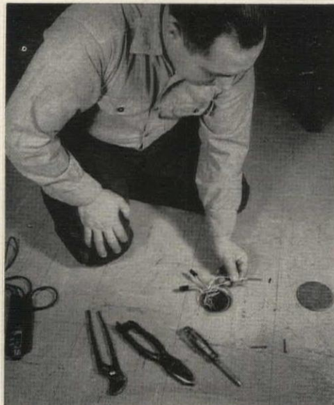
Thermistor probe which senses slab temperature is connected by ordinary electric wires run through conduit beneath slab to remote temperature controllers
