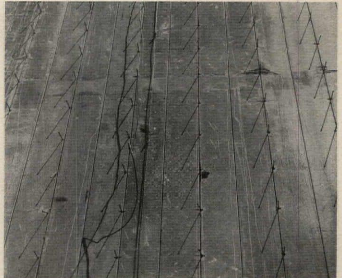
Detail of welded stud bolts to which walers were attached. As walers are removed, bolts are knocked off and scars are subsequently healed by welding
