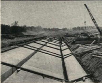
This is the concrete bed on which roof units are cast. Roof units as well as all the other precast structural units are 3,000 p.s.i. lightweight concrete.
