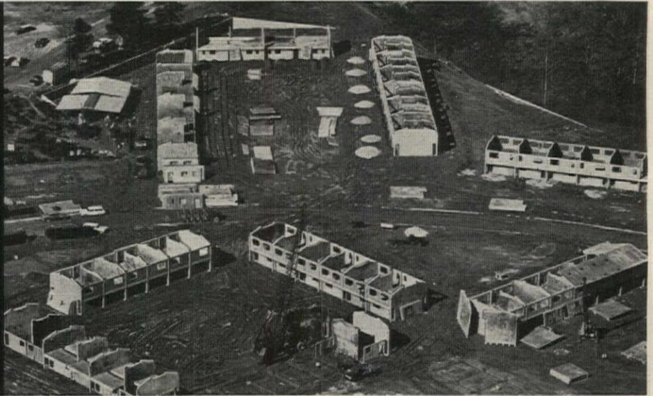
Nine of the 101 buildings in various stages of construction. Entire project covers 80 acres.
