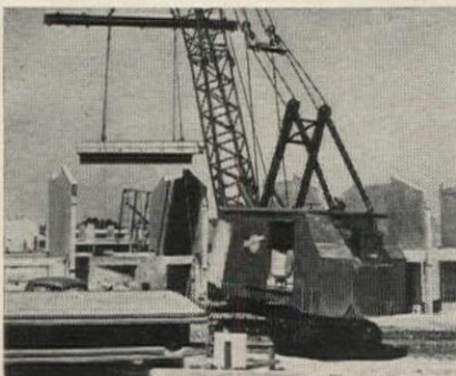
A second floor slab being lowered into place. Supporting beams are cast as an integral part of the slab. Connections are made with weld plates cast in the units.
