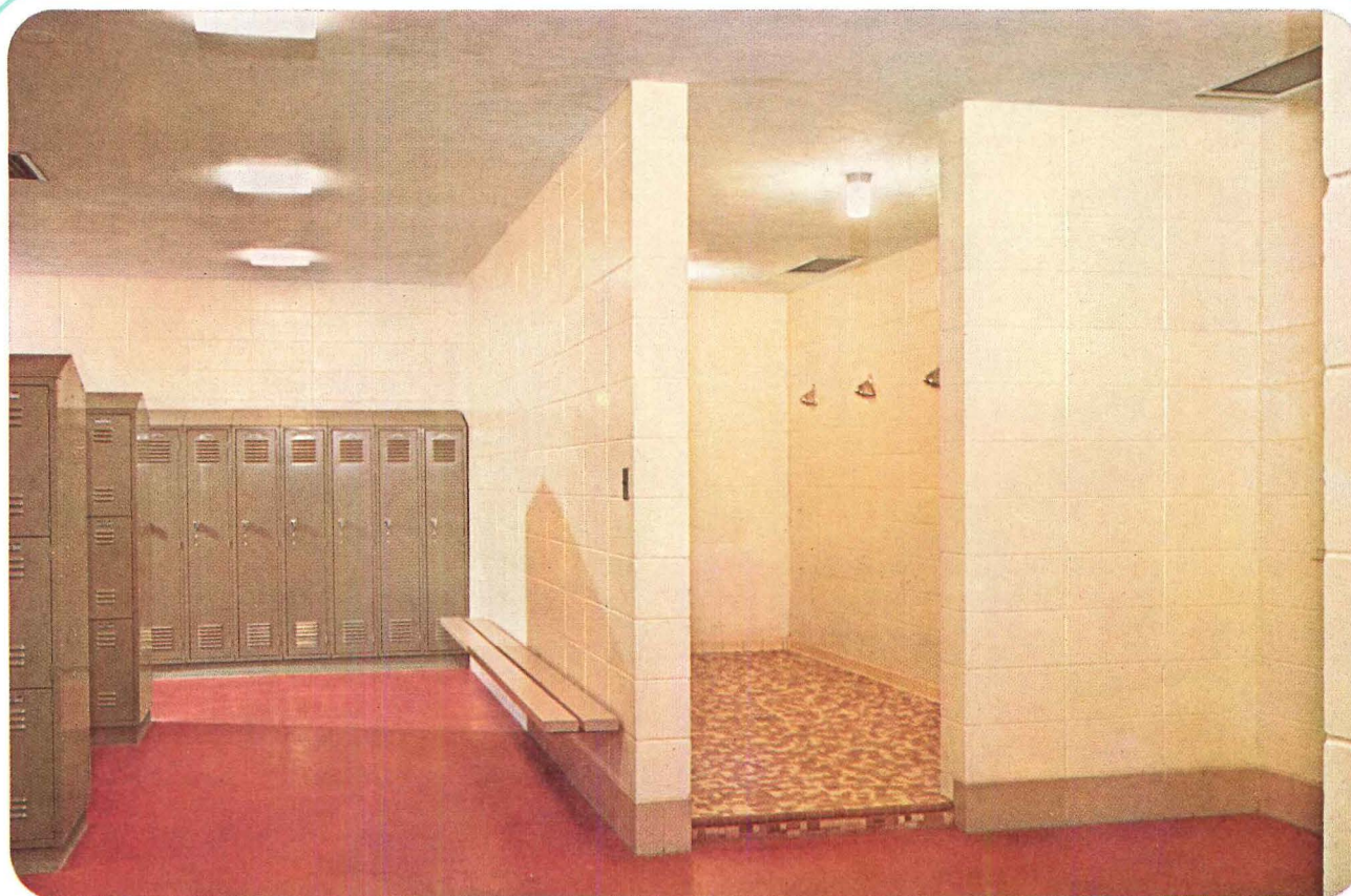
Gertrude Scott Smith School, N. Aurora, Ill.; Architect: Robert F. Mall, Aurora, Ill.; Painting Contractor: Thacker Painting & Decorating Co., Inc., Aurora, Ill.
