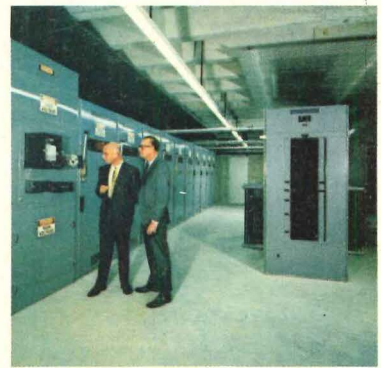
Al Eriqat of Frank L. Hope and Associates, Architects and Engineers, and Ed Butts of Square D examine the main switchgear.
