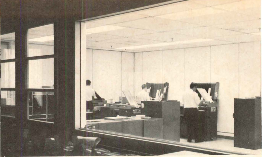
Careful planning is shown by Kerr's data processing room, with underfloor cable space for future equipment. Such rooms are isolated—but with broad expanses of glass for a "wide open" feel. The necessary "micro-climates" are provided by DMS and other Lennox modular systems.
