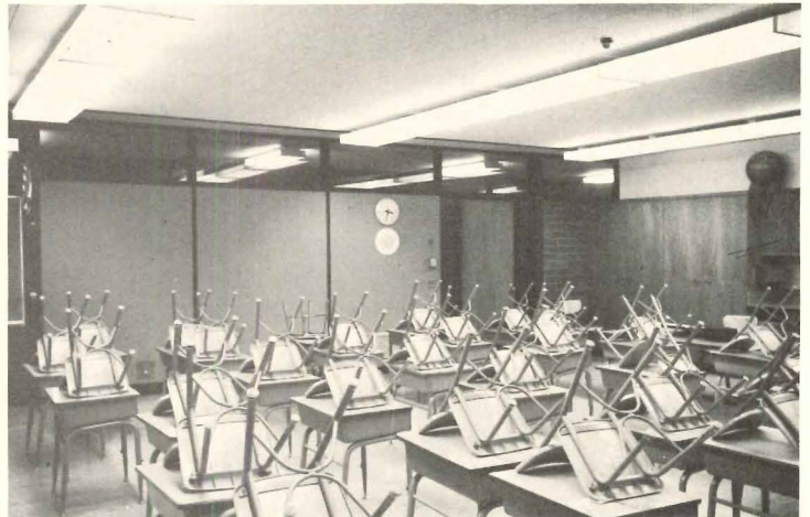
6. Four-lamp, surface-mounted, lens wraparound, 16-in. wide, in continuous rows, 10-ft on center. LEF = 0.165 CRF = 0.749
