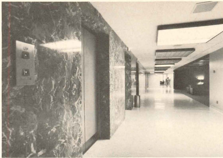
Typical floor area protected by emergency lighting circuits shows one passenger elevator operating; every third fluorescent fixture is lighted.
