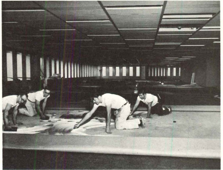
Installers applying adhesive to concrete sub-floor, for direct glue-down installation of double jute-backed carpets in new 64-floor U.S. Steel Building, Pittsburgh.
