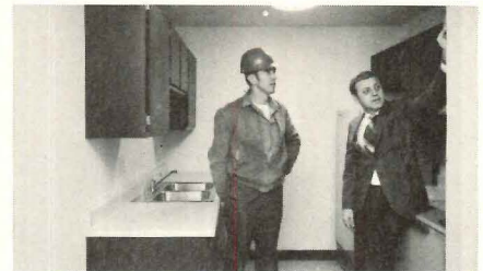
Hide-A-Spray paint dried in two hours. Contractor installed cabinets and floor covering the same day. Walter Scharfe, left, Job Superintendent for Lloyd Construction, commented, “Conventional two-coat paints would have meant a week’s time between painting and any such installation.” PPG Paint Center Manager, Eugene Lee, is shown at right.
