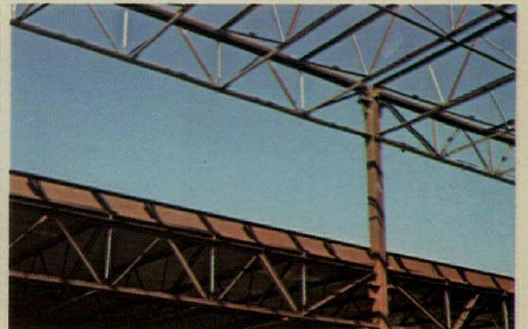
The light weight and simplicity of Vulcraft's steel joists and joist girders make erection fast and easy.
