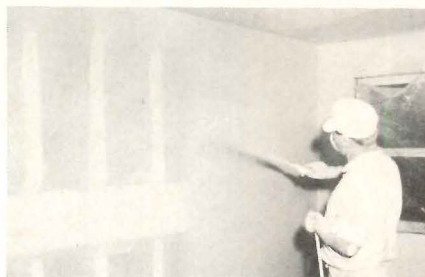
Hide-A-Spray Latex paint completely covered taped and spackled joints in dry-wall in one pass of the airless gun.
