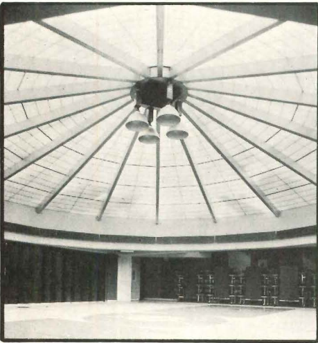
2¾" translucent Kalwall Roof System at Summit School in South Dakota.
