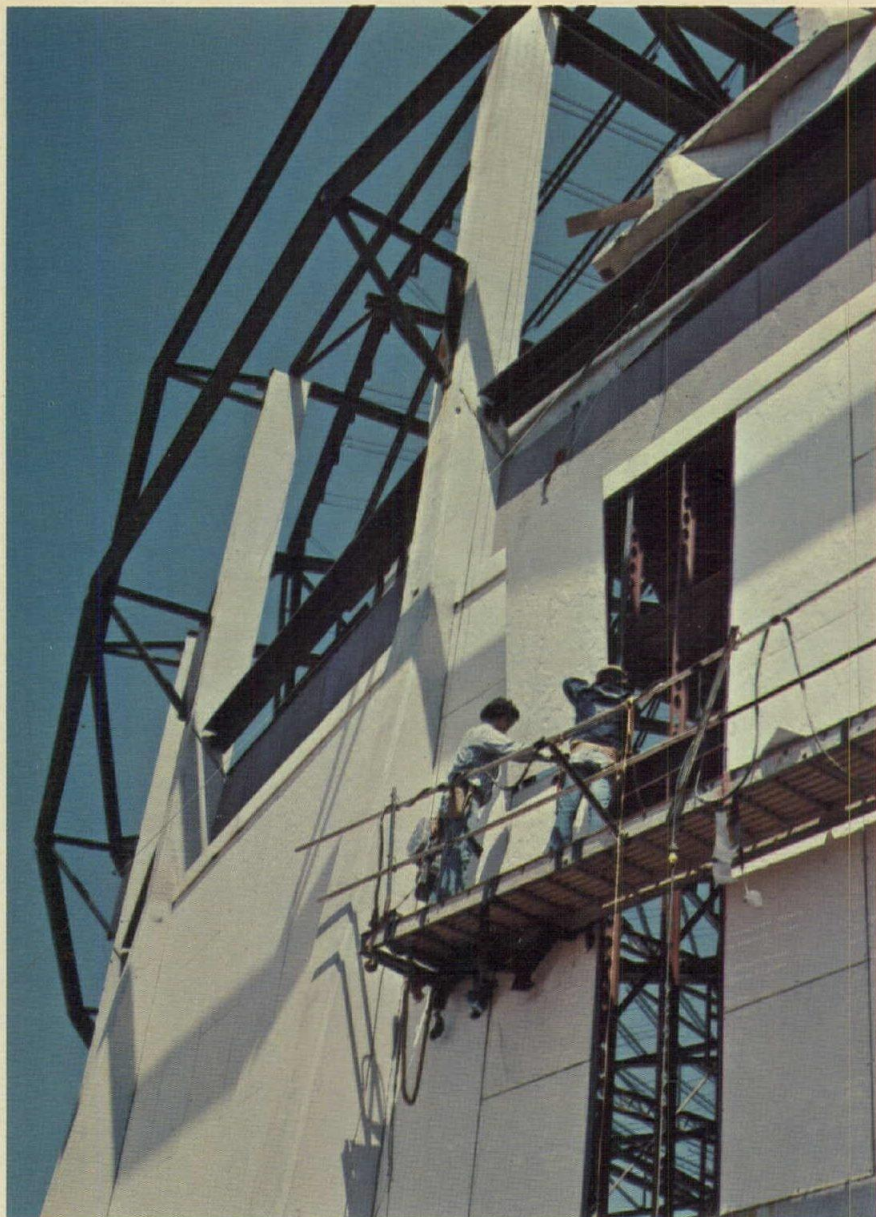
Exterior walls of the new Huntsville, Alabama, Civic Center are J-M Stonehenge® architectural panels secured directly to the steel studs. Here insulation is sprayed on the back of the panels. A combination of hidden and reveal joints was chosen by the architect.
