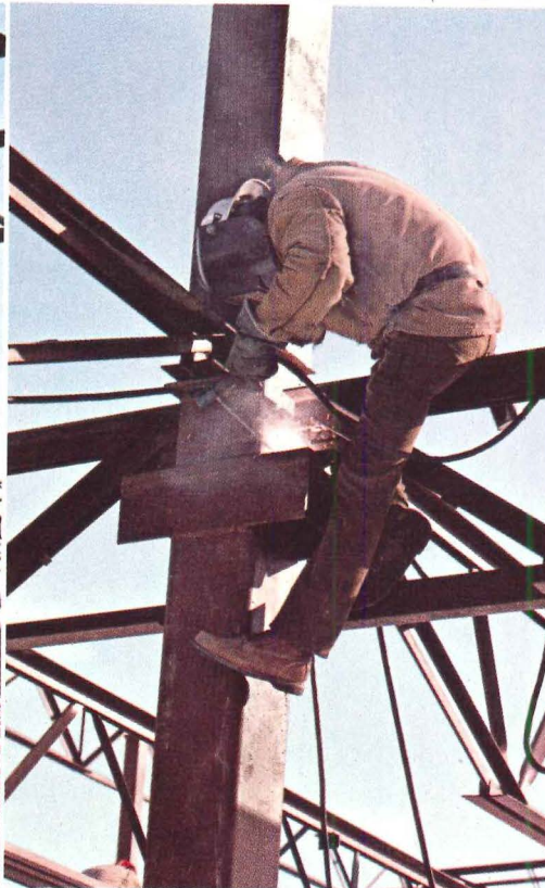
Vulcraft steel joists and joist girders allowed for simple and fast column connections.
