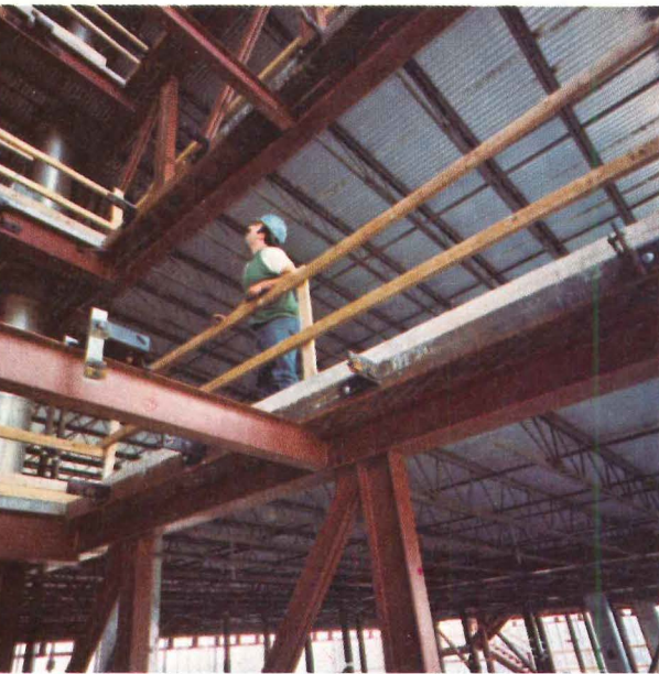
er view during construction shows large, column-free Typical bays measure 53 ft 6 in. by 22 ft. Bethlehem ed 700 tons of structural steel for the project.
