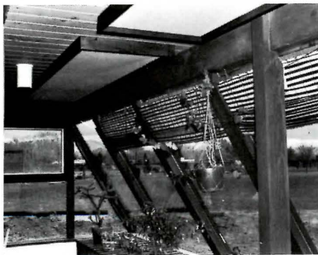
Panels above greenhouse extension
