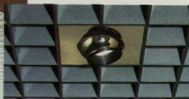
Reflector down lights – polished reflector, mounted for wall washing and overall illumination.
