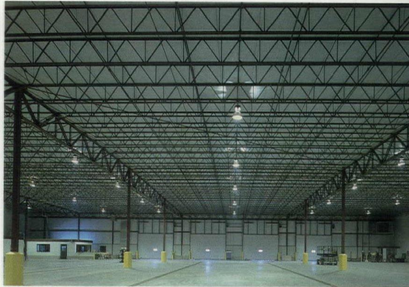
Vulcraft's joists and joist girders also contributed to the cost savings of this job.
