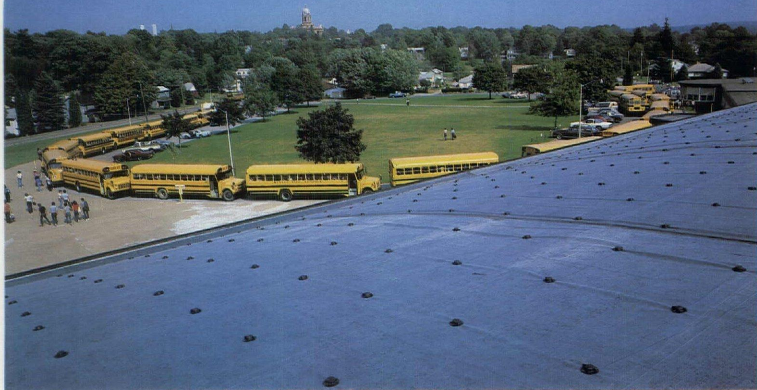
The Mercer Area High School, Mercer, PA Roofing Contractor: J.A. Burns & Sons, Mercer, PA
