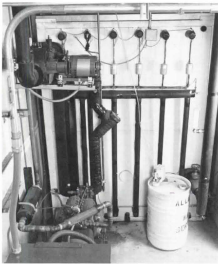
Ice bank and associated mechanical equipment operate with significant reserve capacity in Bank of America installation.
