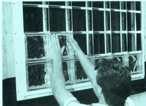
316 Glass-block installation grid. The IBP pre-framed aluminum grid eliminates the need for traditional mortar laying up of all thin-series (3 1/8-in. thick) glass block patterns, making for a much quicker and more uniform installation of walls, skylights, and floors. The biggest standard-size grid is 96- by 144-ins., which can be mullioned together to create larger panels. Perforations in the grid insure good contact of the silicone sealant. Acme Brick Co. Product News continued on page 133
