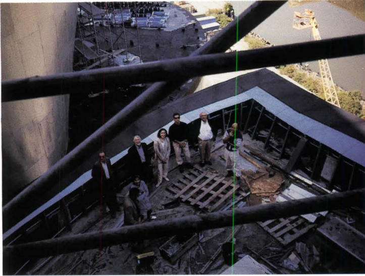
Right: A flooring discussion with, from left to right, Juan Ignacio Vidarte, Luis Rodríguez Llopis, César Caicoya, Vano Haritunians, Edwin Chan, and Gehry. Above: Gehry and colleagues on a lower roof. Far right: The boat-shaped gallery. Opposite: Vidarte, author Karen Stein, and Gehry on a construction tour.
