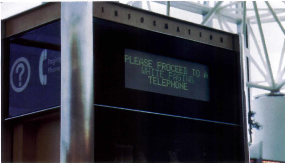
A visual paging system (above), an emergency two-way communica-
