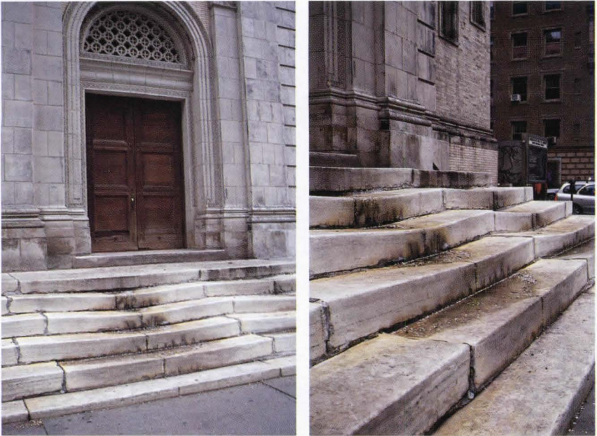
No skateboarders will attempt these stairs, which suffered the effects of weathering and an inadequate substrate. The treads were also not properly angled to prevent ponding.
