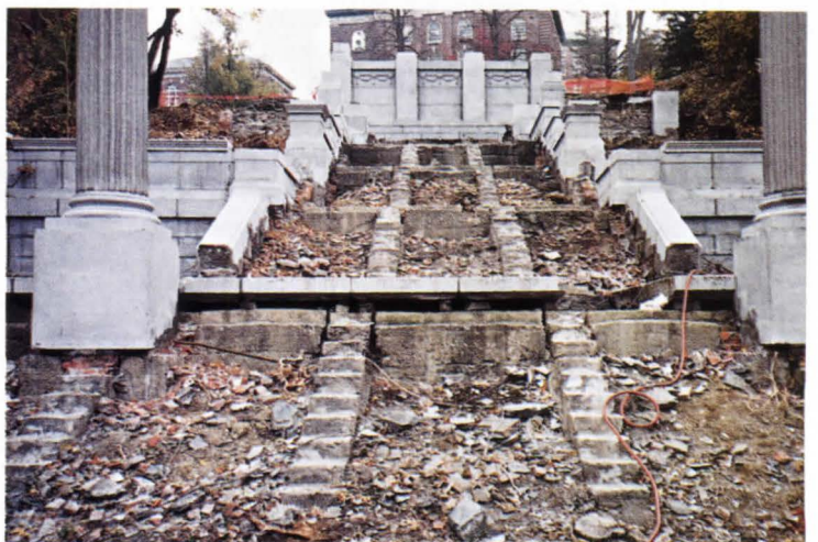
In Troy, N.Y., a 93-year-old stairway leading from the town center to RPI was restored (top) by Architecture Plus after years of neglect (bottom).
