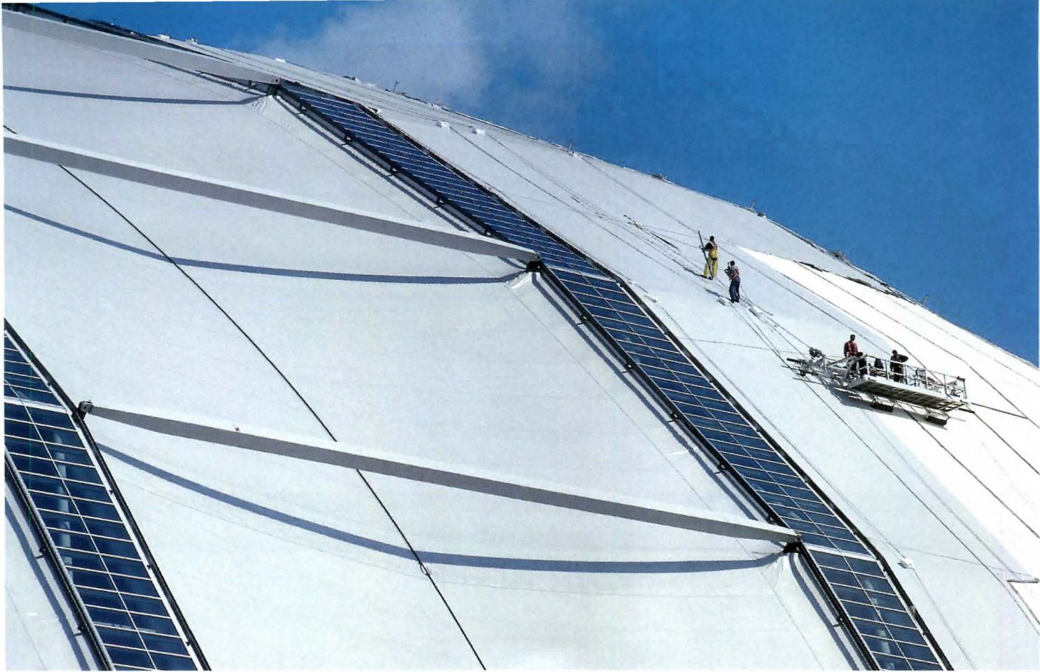
External horizontal props between the top chords of the arches (above) restrain any torsion that might be caused by eccentrically connected membranes. The sliding doors (shown partially opened below)
