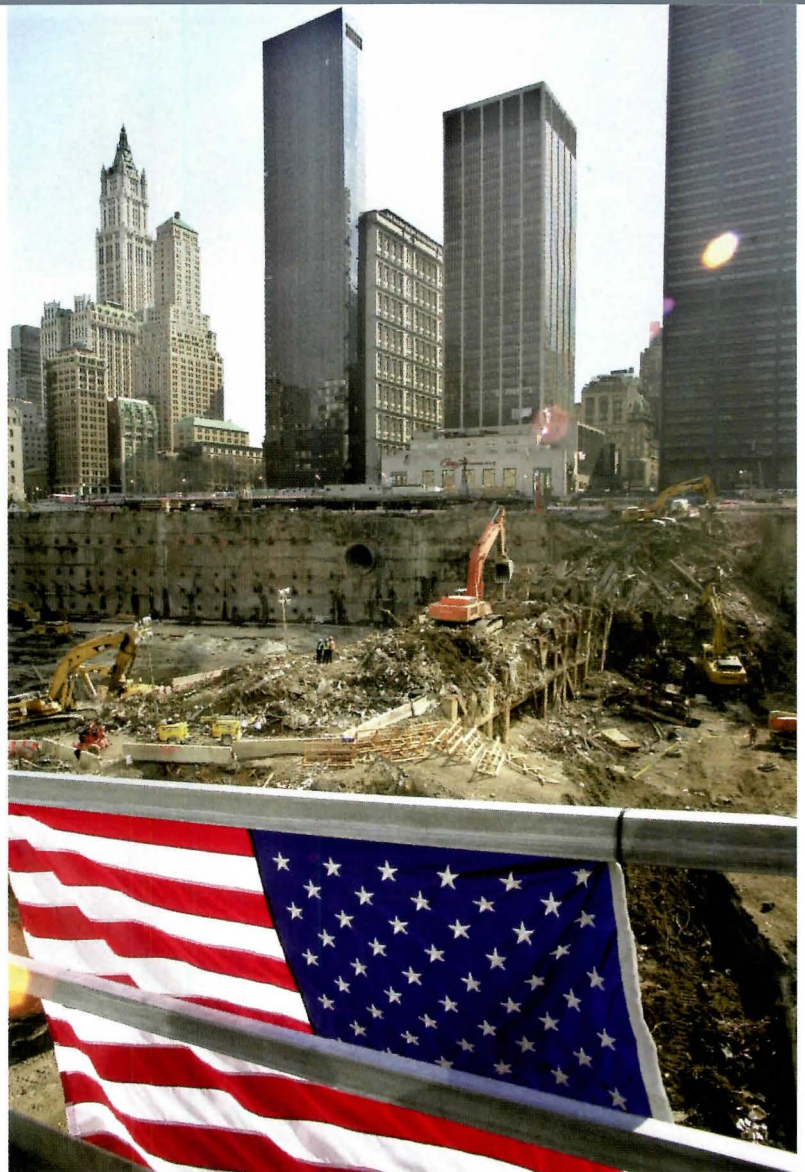
Heavy equipment digs into the last mound of debris at the WTC site in early March.
