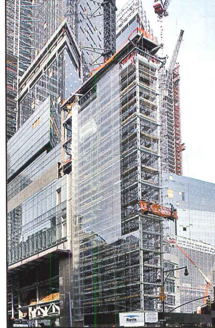
AOL Time Warner, New York City, NY Skidmore, Owings & Merrill LLP, Arch.
