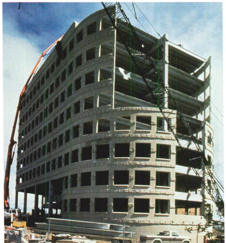
The architectural precast walls of 198 Inverness Drive West, Englewood, CO are the perimeter structural-gravity support for the floors and roof. Architect: POUW & Associates, Inc.
