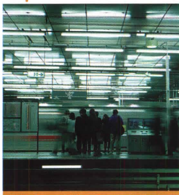
1937 General Electric patents the first practical fluorescent lamp, and introduces them a year later at the World's Fair. Today they're a staple in many office and infrastructure interiors.
