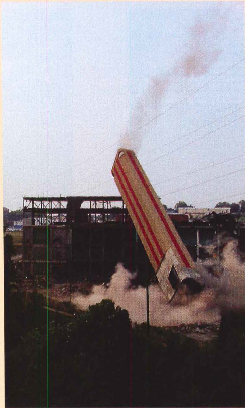
demolition. Electrical equipment from other parts was auctioned off as part of the demolition and dismantling of the entire complex.
