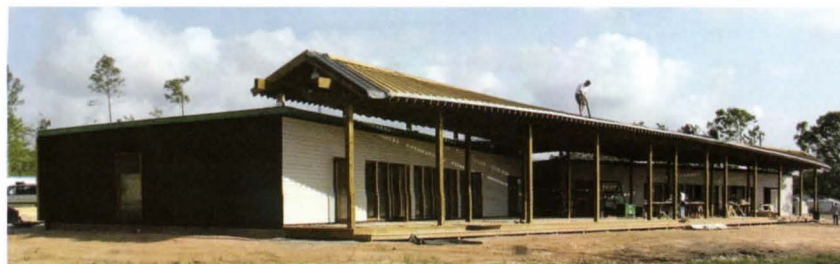
A crew completes work on two SHoP-designed buildings unified by a sculptural canopy.
