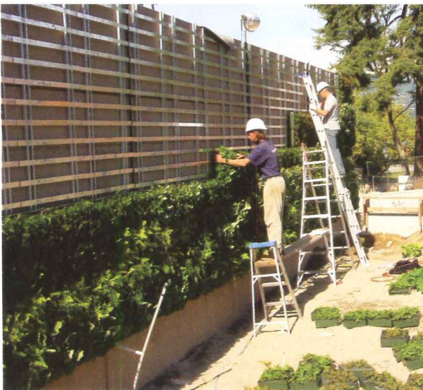
Polypropylene boxes containing pregrown plants such as flowers, mosses, and berries compose the vertical garden at the Vancouver Aquarium. A stainless-steel support grid secures the boxes to the building's structural poured-in-place concrete wall.
