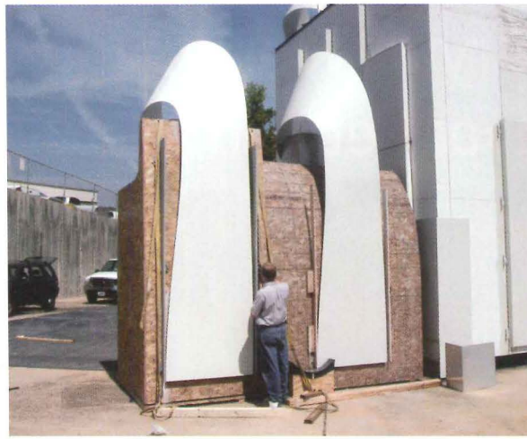
The High's designers built a mock-up of the skylight sunshade to identify any weaknesses inherent in the sail-like shape.
