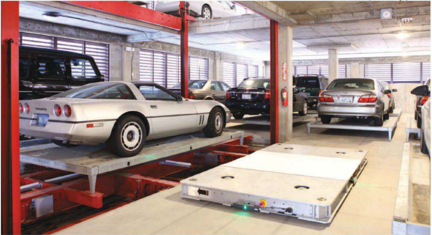
Robots store and retrieve cars on steel trays in this latest-generation automated parking system in Crystal Springs Resort, Hardyston, New Jersey.
