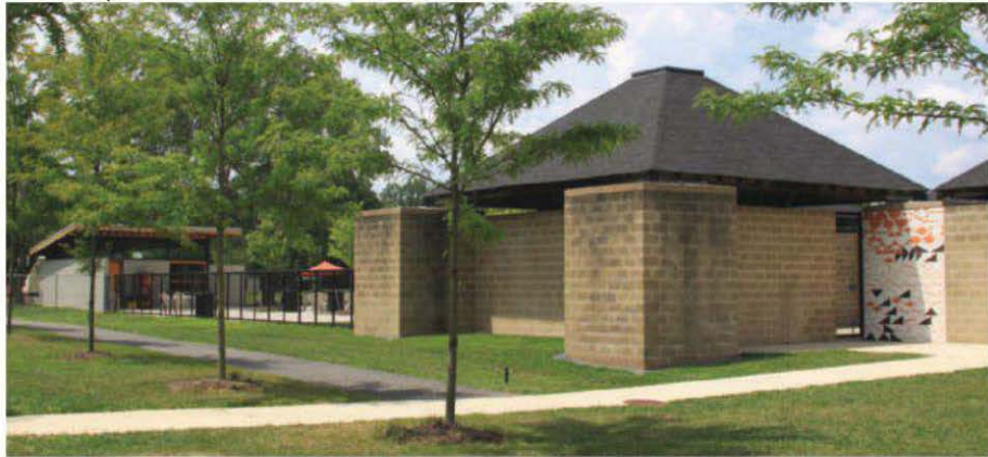
New Jersey's Louis I. Kahn Trenton Bath House uses a unitized flashing system on two new walls.
