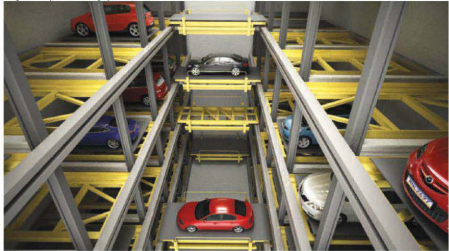
Second-generation “mono-path” shuttle and lift system
